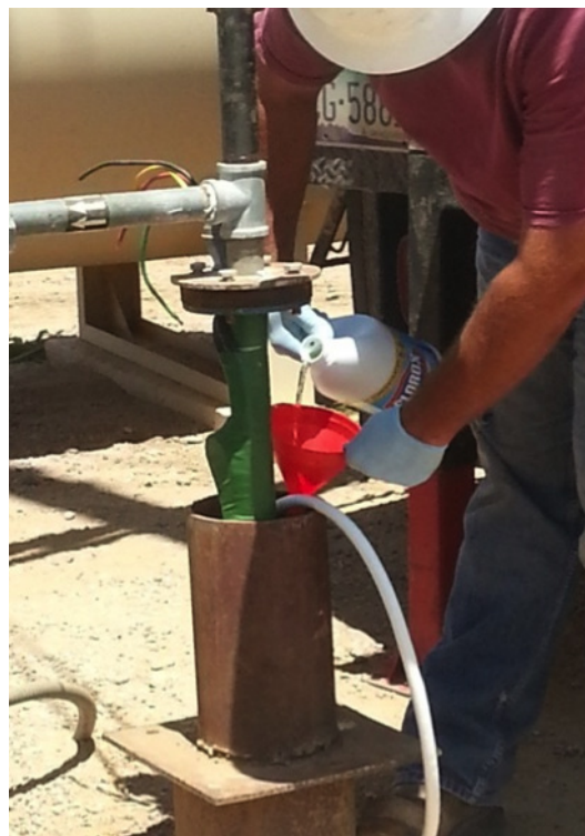
Figure 9. Contractor chlorinating a well. Note safety equipment and water circulation hose through the opened well seal, something most well owners cannot do themselves. Photo by G. Hix.
